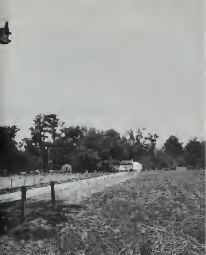
Typical REA-financed construction on the farm of T. L. Burgess in Clarendon County, S.C. The pole is used also by the telephone cooperative.
